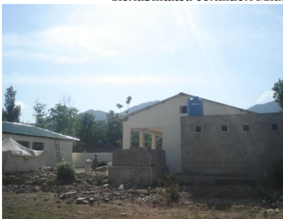
Figure 10. Condition of Exterior Wall-1
