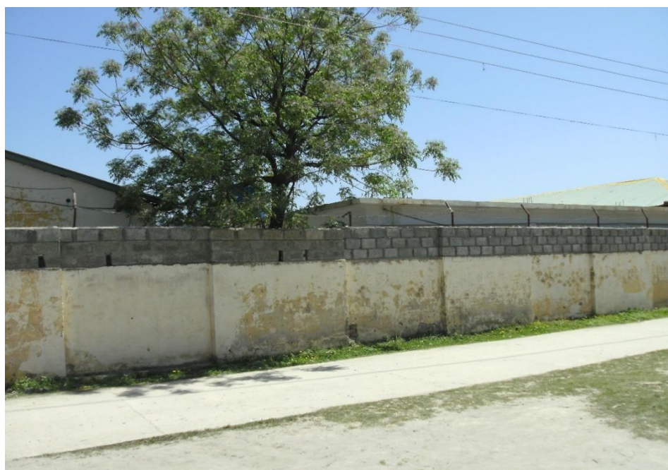
Figure 23. Boundary wall height extension for safety from intruders.
