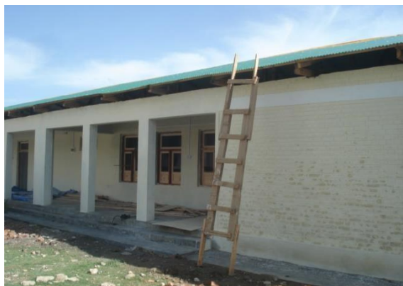
Figure 15. Condition of Exterior Wall
