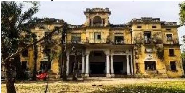
Figure 2: Façade, existing visual condition
